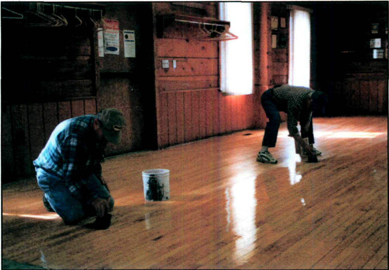
Gene Schacht and Bob Vincent are shown putting the finishing touches on the dance floor.
